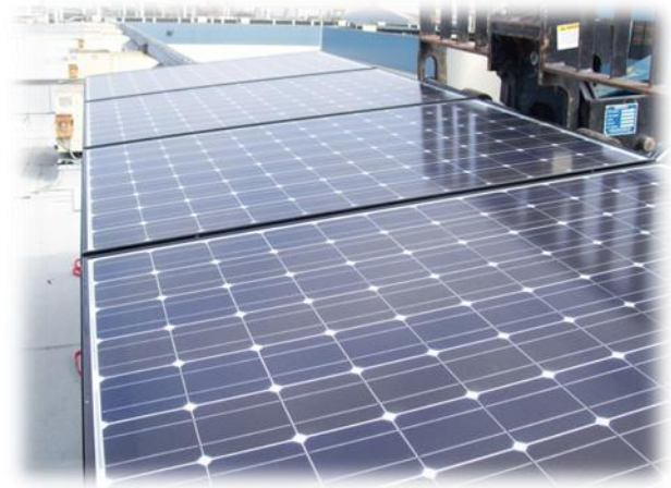
The newly installed solar panels on the rooftop of UpTick's San Francisco headquarters.
